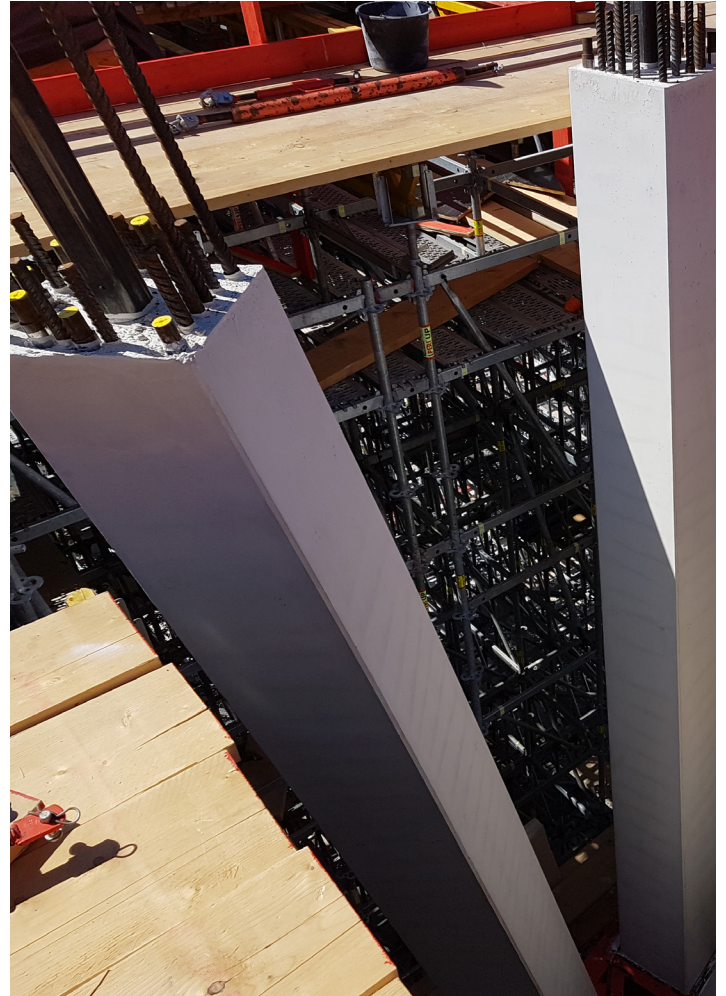
The head point of the tree support with connection reinforcement for the floor slab above the foyer. (©Wulle Lichti Walz)
